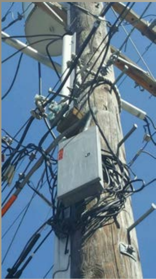
Jointly owned Pole with Equipment tied by Rope and Obstructed Climbing Space, Photo by Catherine Sandoval, March 2018
