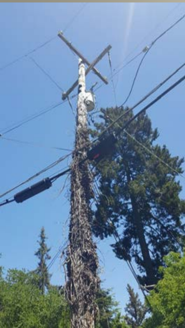
Photo: Tier 3 High Wildfire Danger Area, Los Gatos, CA, Utility pole wrapped with dead vegetation, Photo by Prof. Catherine Sandoval, May 2019
