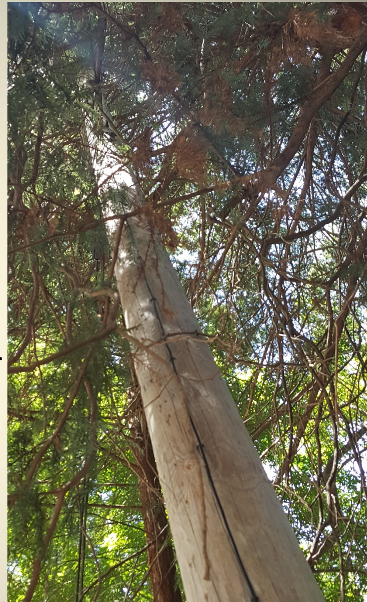
Tier 3 High Wildfire Danger Area Utility pole trapped in vegetation Photo by Prof. Sandoval, May 2019
