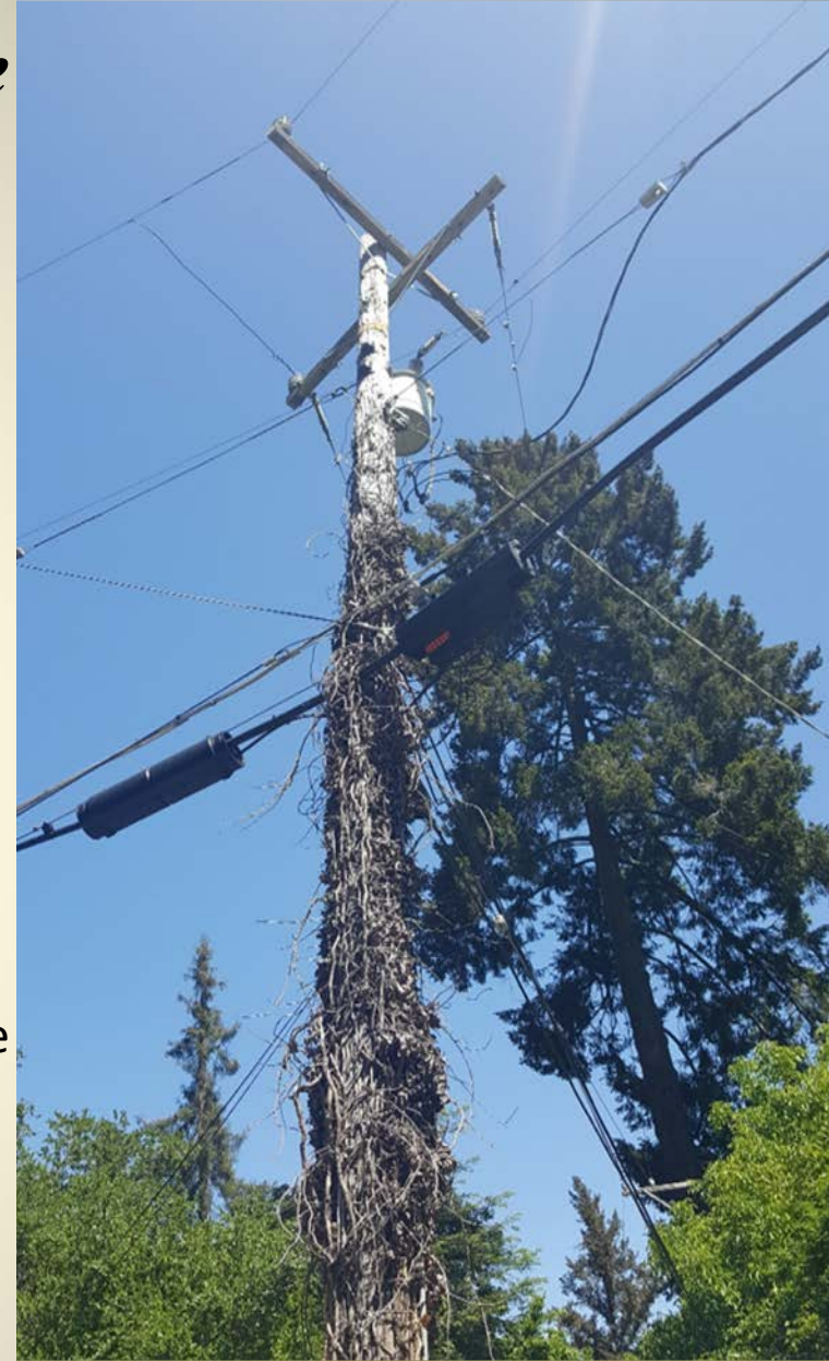
Tier 3 High Wildfire Danger Area Utility pole trapped in vegetation Photo by Prof. Sandoval, May 2019
