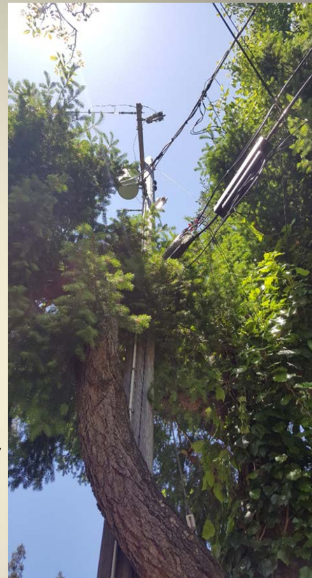
Vegetation too close to pole and wires in Tier 3 High Wildfire Danger Zone, Los Gatos, CA, Photo by Prof. Catherine Sandoval
