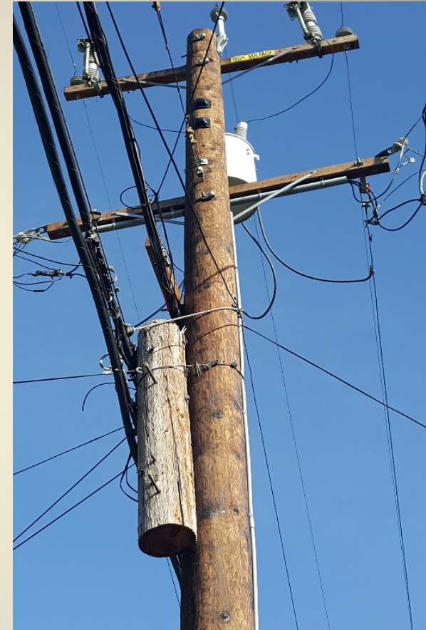
Photo: “Peg” Old pole tied to new pole by rope, San Jose, CA, Photo by Prof. Catherine Sandoval, April 2018
