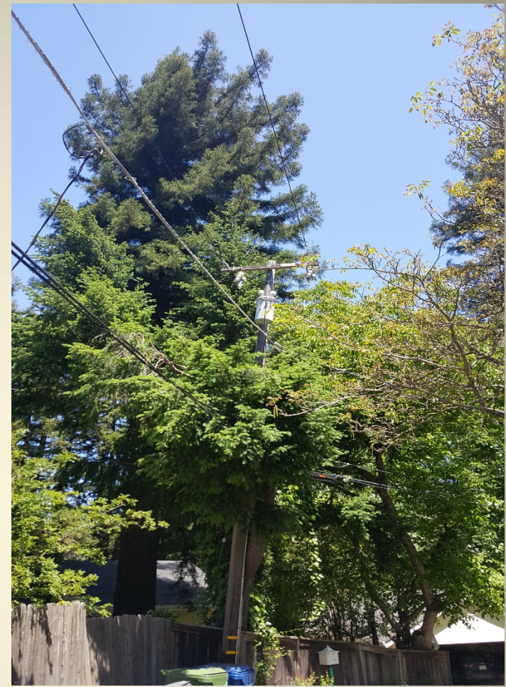
Tier 3 High Wildfire Danger Area, Los Gatos, CA, Overgrown vegetation compromises safety and utility pole access Photo by Prof. Catherine Sandoval, May 2019
